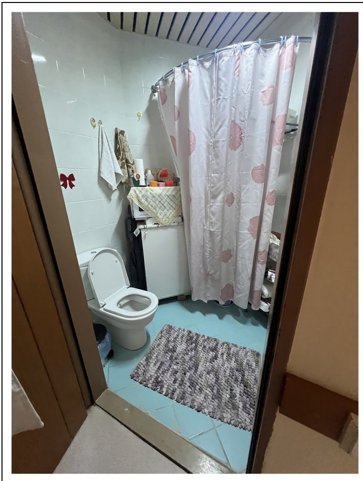
Figure 9. Low safety features: Lack of nonslip materials and grab bars.
